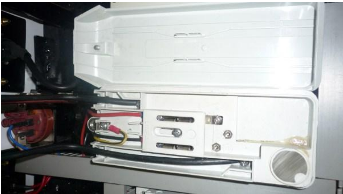
Cover of the HV transformer removed, showing interlock's and wiring. Notice the important safety earth.
