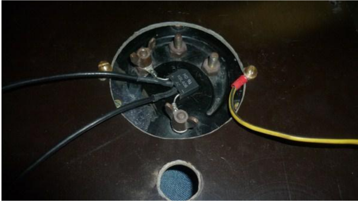
Underside of the ammeter. Notice the bridge for AC current measurement.
