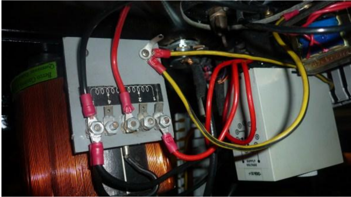
Some of the wiring around the variac. The grey module is an electronic timer that has subsequently been swapped out for a mechanical unit, as its noise immunity was not high enough. All exposed metal is properly grounded to drain off static.
