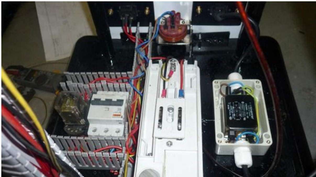
Components being fitted to the base. At the rear is the pressure emergency off switch. RHS is the EMI mains filter. Centre is the neon sign transformer. LHS is the main control relay, and mains isolator. All wiring is inside slotted trunking to neaten it up.
