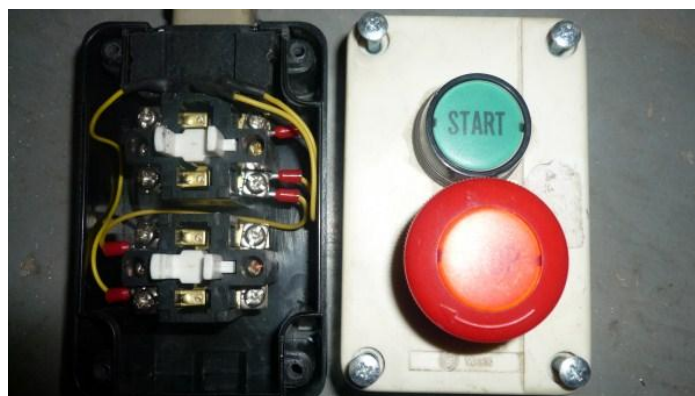
Wiring of the remote control pendant.
